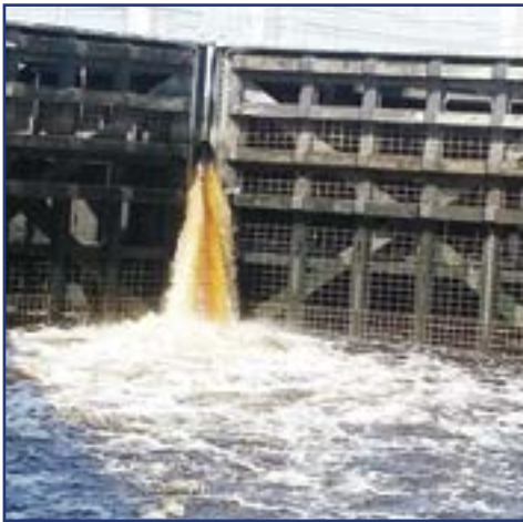
Opening of one of the five locks along The Okeechobee Waterway that extends from the Atlantic Ocean at Stuart Florida, to the Gulf of Mexico at Ft. Myers.
